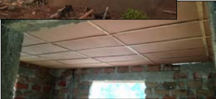
Installing ceiling tiles; we are praying the lodge is complete before November in order to house brethren, both local and international.
